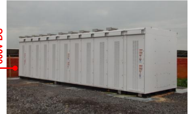
2 x 1MWh DC System
